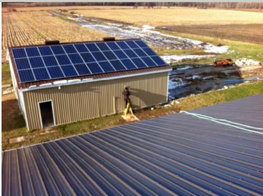
PV Energy System - 9KW on Building 1
