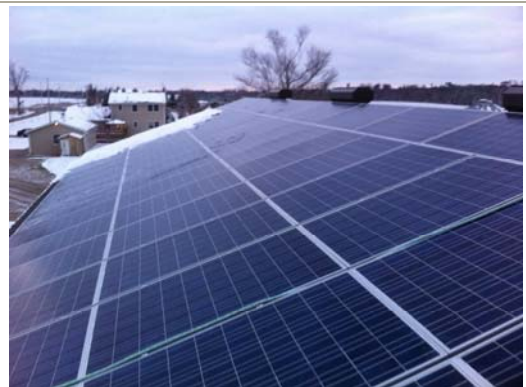
PV Energy System - 11KW on Building 2
